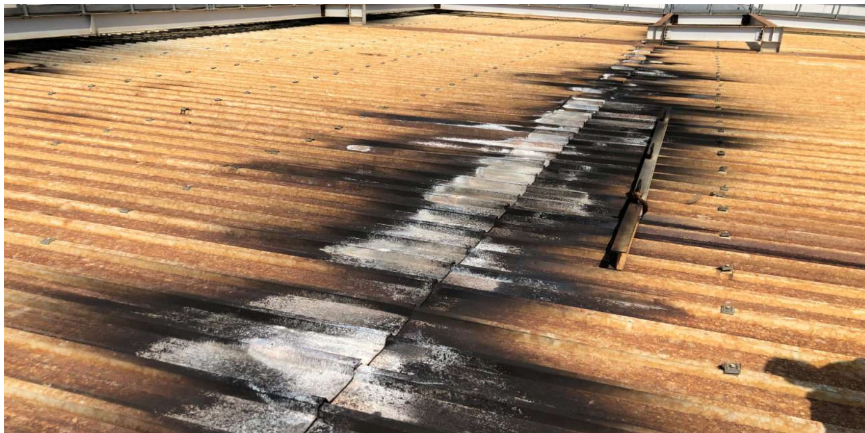
Figure-15 Corrugated sheets at roof is badly burnt at several location which makes the structural adequacy of corrugated sheets doubtful.
