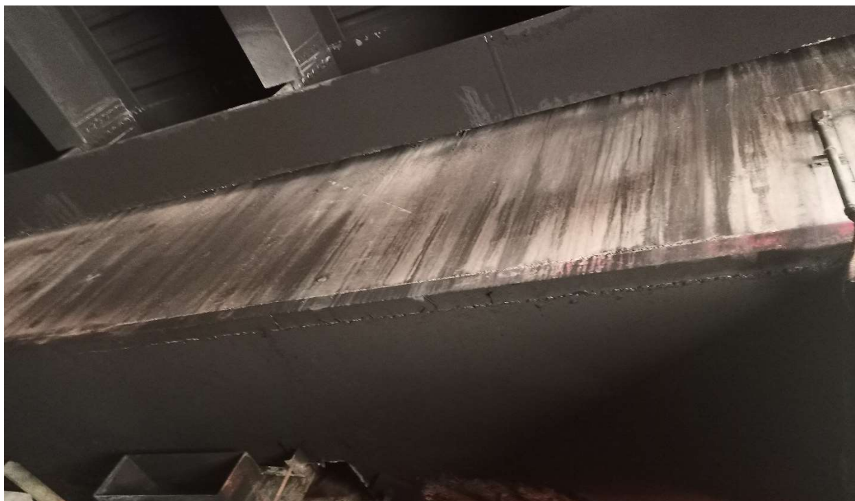
Figure-7 Another Bracing Beam at Level-01 is smoky underneath without impairing the beam physically and structurally.
