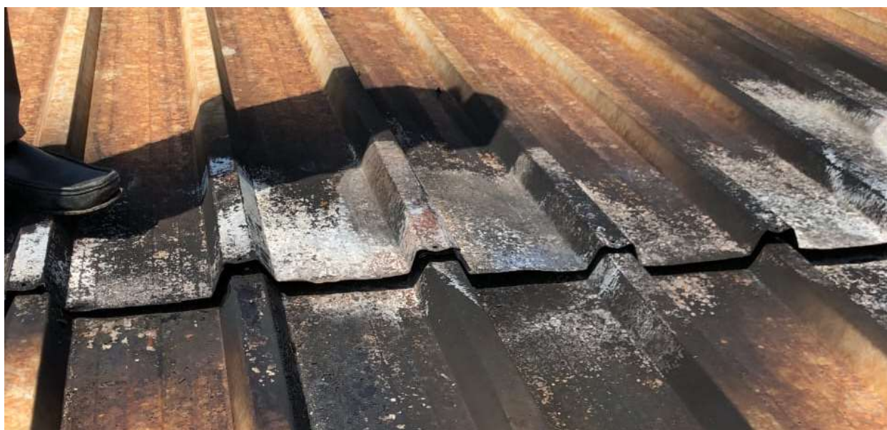
Figure-16 Absence of rivets/screws has enlarged the gap at the sheets overlapping location which ultimately results in leakage of rain water down the Stream Turbine Hall.
