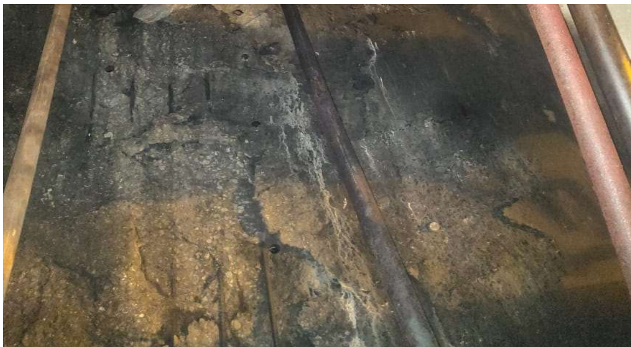
Figure-6 Shear Reinforcement of Bracing Beam at Level-01 is exposed due to fire.
