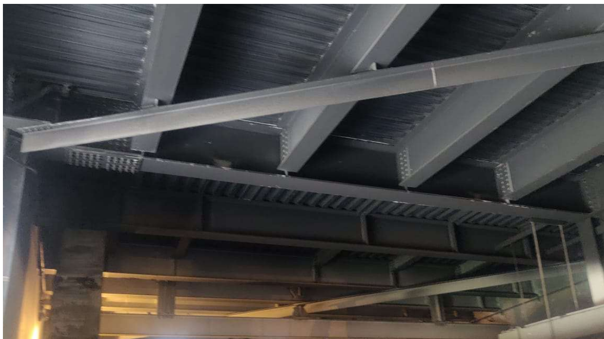
Figure-11 All Steel beams at Level-01 are smoky due to fire incident without adversely affecting the structural strength.
