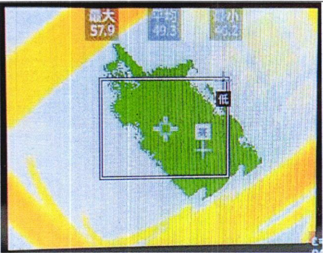
Temperature at stator bottom(TE)
