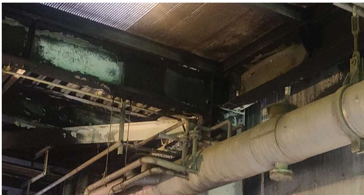
Figure-12 All Steel beams at Level-01 are smoky due to fire incident without adversely affecting the structural strength. Furthermore, the paint of almost all steel beams is deteriorated.
