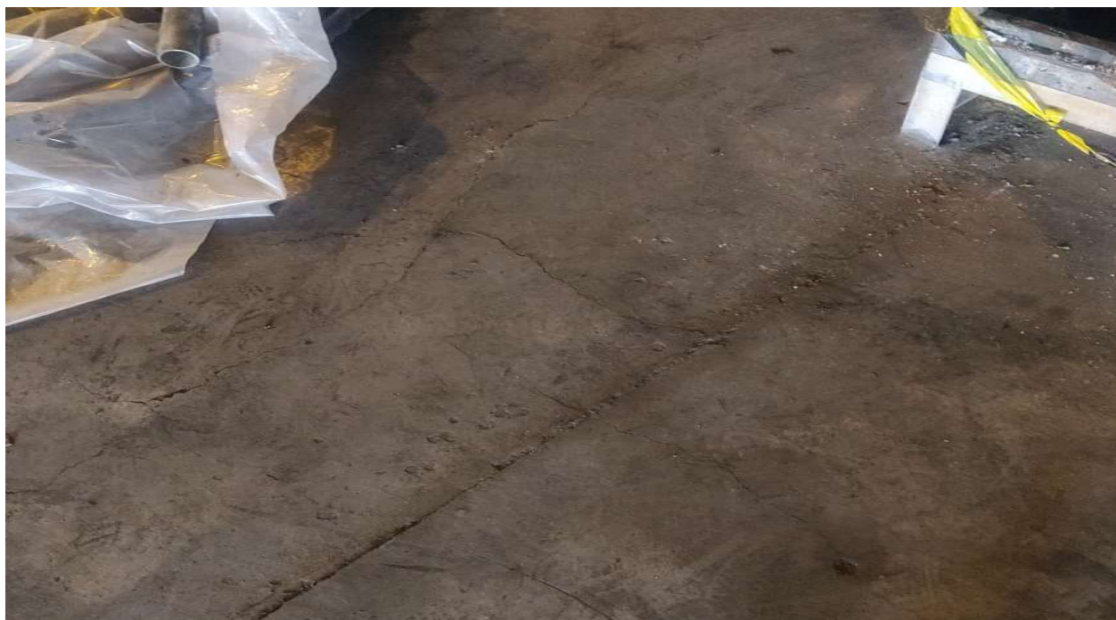
Figure-3 Level-2 Concrete topping which was casted above the ST foundation/beam has been severely damaged/cracked at the right side of ST-16.
