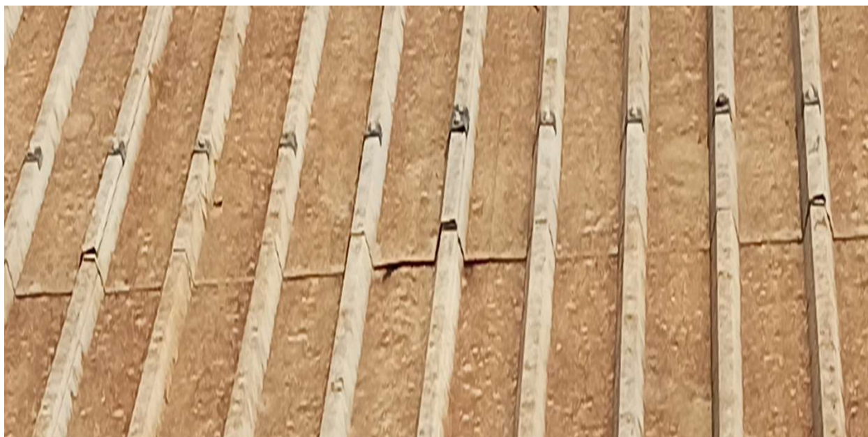
Figure-18 Absence of rivets/screws and water proofing paint at almost all the roof has substantially deteriorated the corrugated sheet
