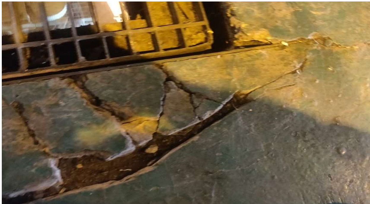
Figure-1 Level-2 Floor Concrete has been damaged at various areas specially near the manhole and edges
