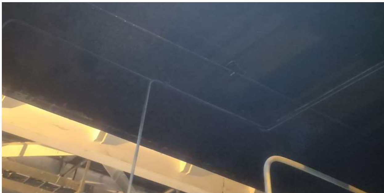
Figure-8 Another Bracing Beam at Level-01 is smoky underneath without impairing the beam physically and structurally.
