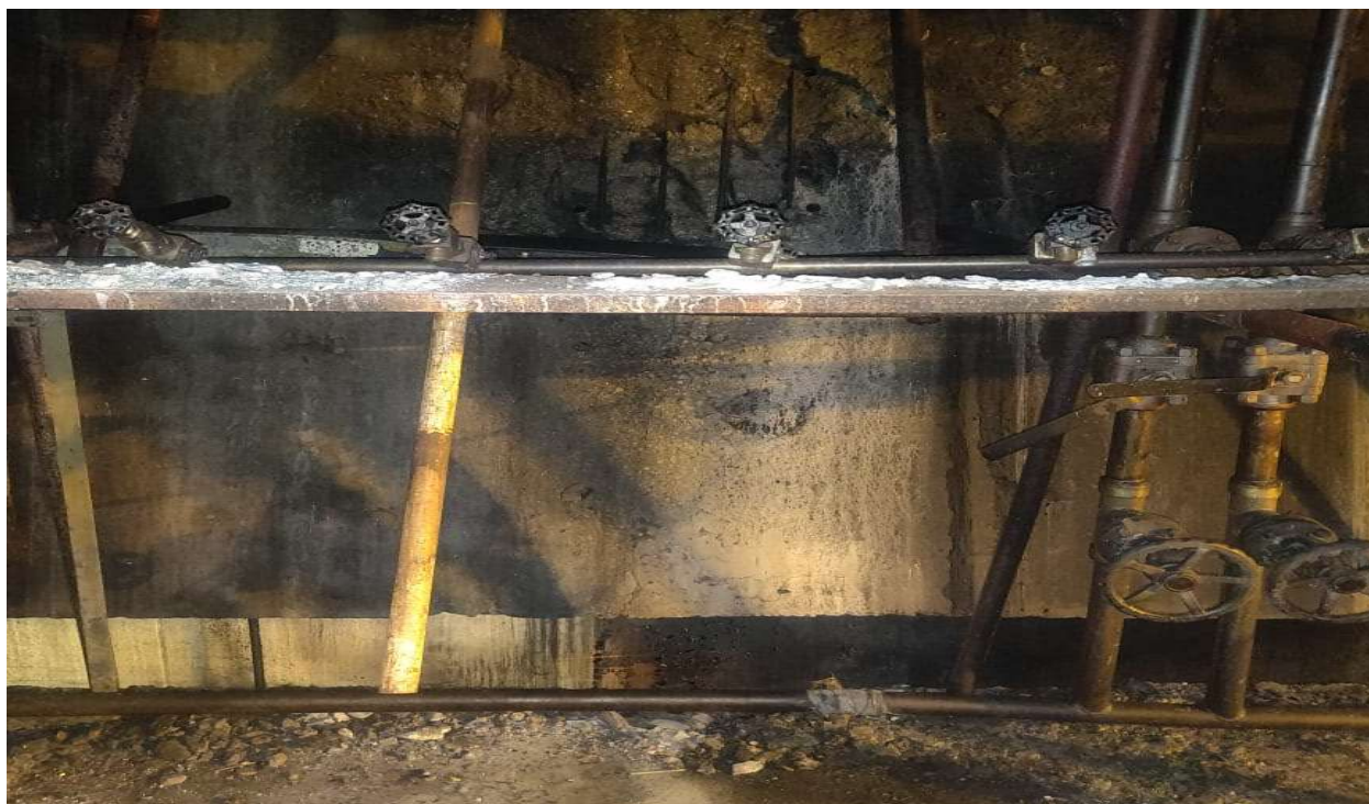
Figure-5 Bracing Beam at Level-01 is severely damaged nearly in the mid-span due to inherent fire passage at the bottom
