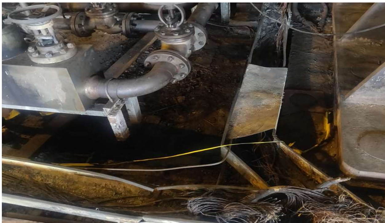
Figure-4 Level-2 Concrete topping underneath ST-16 is severely damaged.
