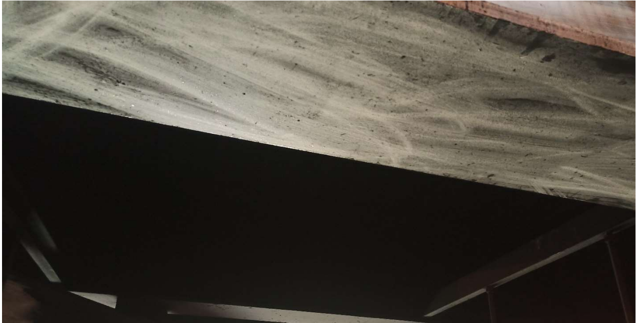
Figure-13 Smoke deposits from the steel beams were cleaned manually, and inherent color of steel beam can be seen.
