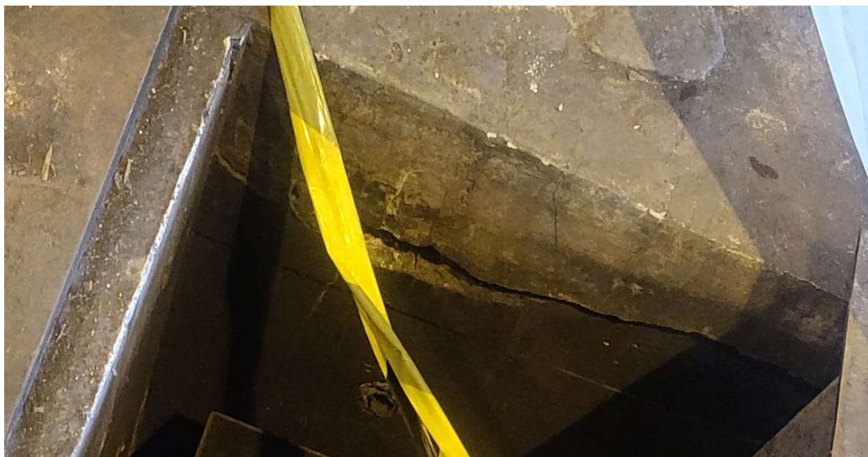
Figure-2 Level-2 Concrete topping which was casted above the ST foundation/beam has been severely damaged/cracked at the right side of ST-16.
