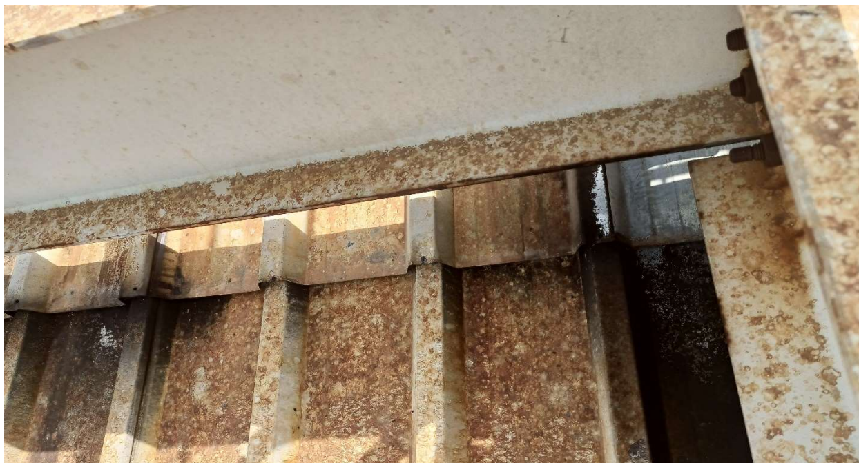
Figure-17 Absence of rivets/screws and water proofing paint at almost all the roof has substantially deteriorated the corrugated sheet.
